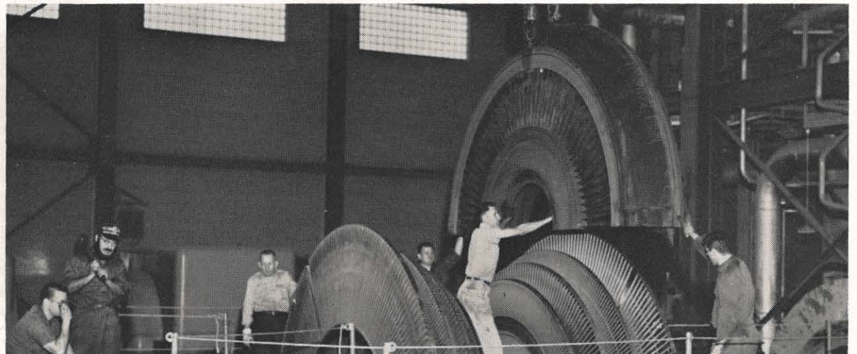
More than a mile of tubing was replaced in the course of major overhaul work done on Kanawha River plant's Unit No. 1 in May and June. The complete secondary superheater was resupported, and the entire
