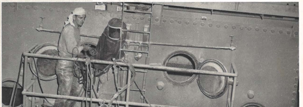
Clinch River plant's No. 2 Unit was out of service for scheduled maintenance work from June 29 through July 7. In the course of the work some major projects were completed. They included relining the ash hoppers with an eight-inch refractory wall, washing and cleaning air pre-heaters, and repairing the unit's steam condenser waterbox. In this picture George Abshire, maintenance man, is assisting in the work of sandblasting the surface of Unit 2 steam condenser prior to painting.
