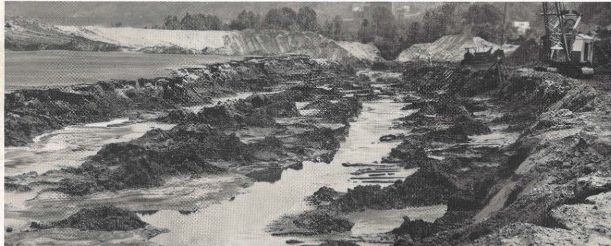
It may look like the surface of the moon, but it isn't. This is a shot of the work being done to create additional storage space for fly ash at Glen Lyn plant. The dike wall is being increased another ten feet.
