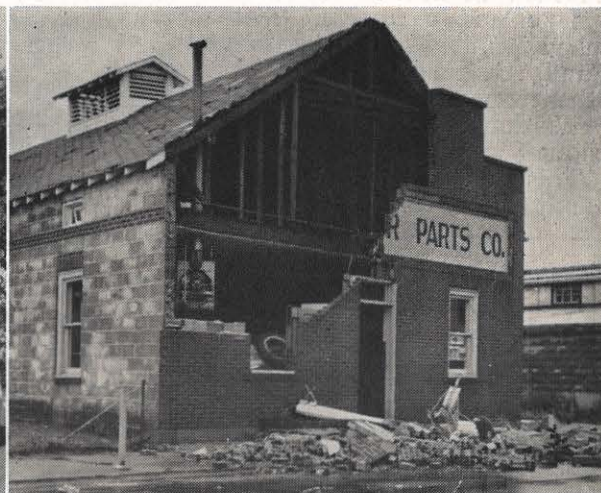
At right, an auto parts firm is minus the front of its building, ripped away by the high winds. Damage like this was a common sight in Ravenswood after the storm. (Photos by Joe Short, Ravenswood News.)
