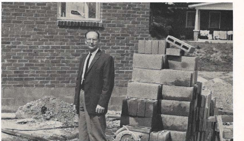
M. E. Rich stands before the infirmary-dispensary now under construction at Camp Joy.
