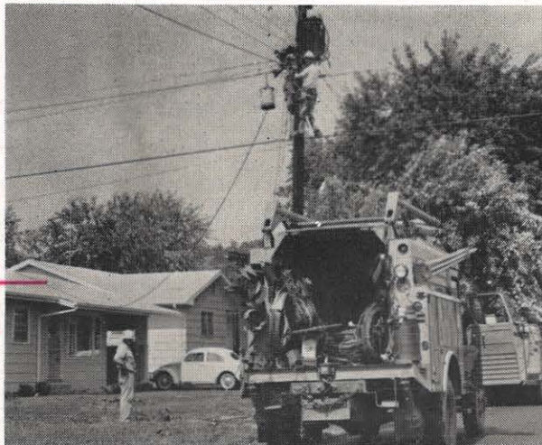
The Ripley line crew restores service and replaces damaged wires in the aftermath of the sudden storm which shook Ravenswood in July. Six hundred customers were out of power as a result of storm damage.
