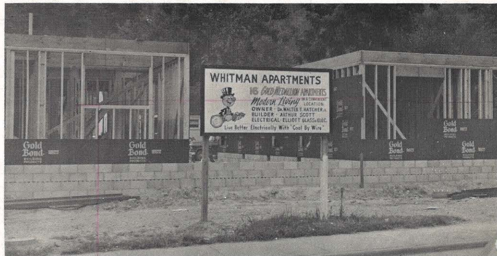
Reddy Kilowatt and his Gold Medallion key identify Pikeville's newest apartment development as featuring the best in electrical living.
