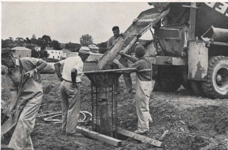
Leroy Pothress, Bluefield division civil engineer, watches the progress of concrete pouring at the site of the Princeton Project Decision building. Because of the nature of the soil at the site, concrete cassions had to be poured to support the building's foundations. There are 80 cassions; they average about 17 feet in length with a three-foot concrete bell at the bottom. Diameter is two feet.
