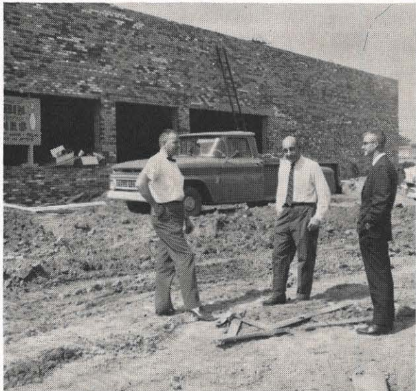
Two new all-electric 24-lane bowling alleys are going up in the Charleston area, scheduled for completion next month. Each has 40 tons of heat pump equipment, plus electric cooking, water-heating, and pin-spotting facilities. In the picture at left, Stuart Foehr, left, and Ranny Woodyard, right, division commercial
