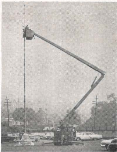
There was no brush with a handle long enough to do the job, so when the 65-foot flagpole at Glen Lyn needed painting, they got a bucket truck, and sent up W. B. Basham and W. F. Cohran. Both are in the system transmission department.
