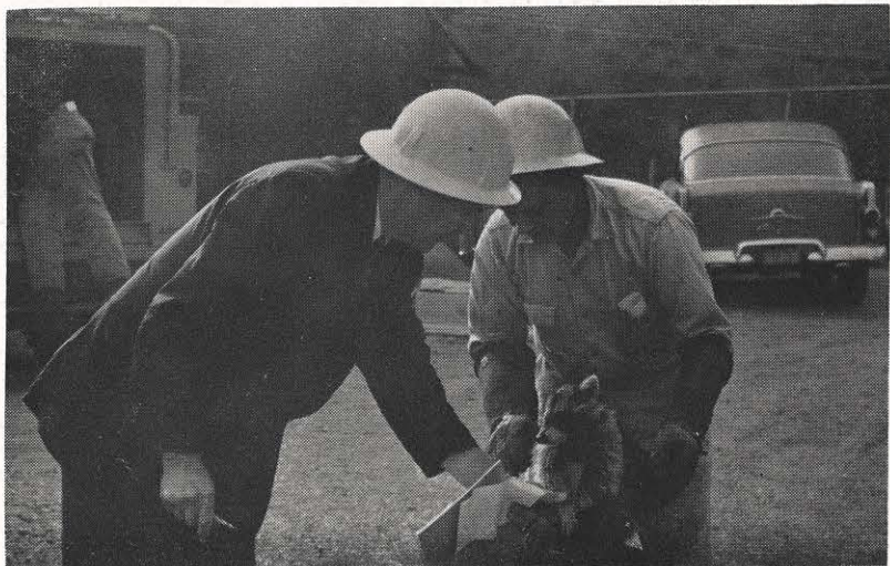
Now it's raccoons. Customers in the Belfry section reported they were out of power. J. R. Hartzog, meter service foreman in Williamson, and Ira Conn, meter serviceman, went out to have a look. And there, resting permanently on a transformer, was a 20-pound coon. He had apparently climbed a pole and touched a wire and thus set off all the trouble. The two investigators said it was the first time they have traced trouble to a coon. Snakes, birds, squirrels, and cats, yes; but coons—no. In the picture, enacting the crime, are Mr. Hartzog, left, and Mr. Conn.
