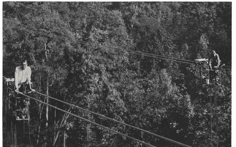
Final work on the Kanawha-Cloverdale 345-kv line was being completed near Kanawha when this picture was made. In this photograph, taken by J. C. Burnette, safety supervisor at Kanawha River plant, two workmen are installing mid-span spacers, designed to keep conductors from making contact with each other. They are riding gasoline buggies that carry them from span to span along the conductor, sometimes as high as 1,000 feet above solid ground. The work here is "only" 100 feet up.
