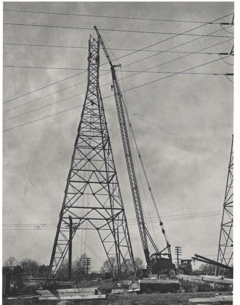
A tall crane, resting on a special platform, adds ten feet to the height of a 138,000-volt tower, which had to be re-located because of highway work.
