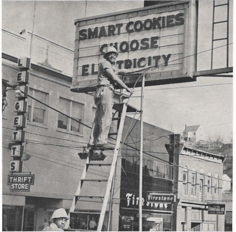
What is believed to be Appalachian's one and only marquee sign is on the Bluefield office building. Twice each week a new sign, either advertising electricity or promoting certain civic campaigns such as the United Fund, goes up. There are times when it's tough to think up a new one, says the sign's resident author, Ira Henderson; he welcomes suggestions. The sign has three lines of 13 characters each. Some of the most recent attention-getting signs have been "Home on the Electric Range," "Go Fly A Kite—Away From Power Lines," and "Electric Hot Water For April Showers." Garland Morrison, top, and John Hurt are shown changing the sign.
