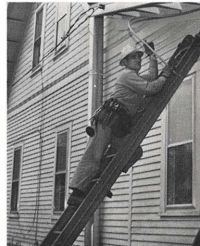
The wrong way: H. D. Morrison, Huntington meter service helper, picked a ladder too long for the job, and leaves the man on it in an awkward position to do his work.
