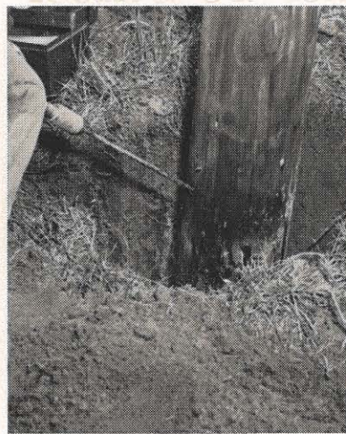
quarter-inch of preservative. The bandage covers 20 inches of the pole and is stapled in place. The
