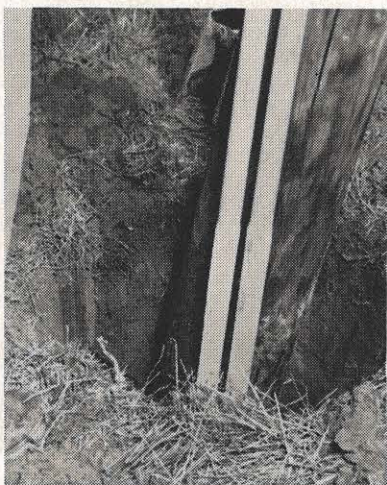
The pole is excavated 18 inches below the groundline. Then it is inspected and cleaned of dirt and
