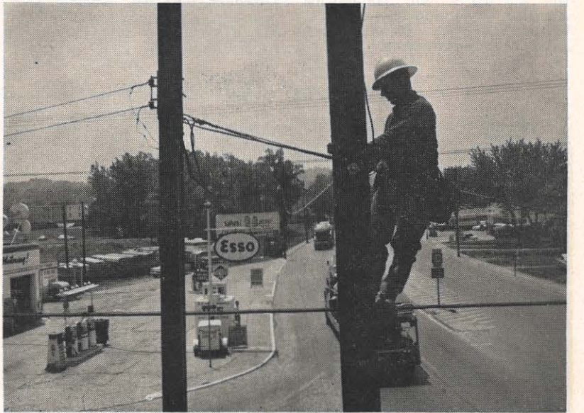
High above McCorkle Avenue in South Charleston, John Moss, lineman, works on transferring wiring to a new pole as part of a new street lighting project. In the course of the work 123 21,000-lumen lights will be installed and 105 new poles set. The entire job will be finished by June 30, and will bring the average illumination level along the street to recommended levels.
