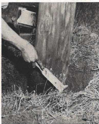
loose wood. A test bore for inner decay is made at the groundline. A paper bandage is coated with a
