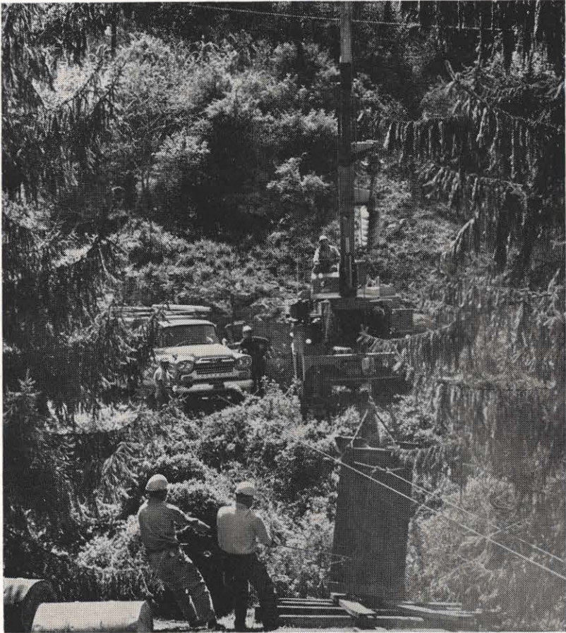
R. R. Jones's substation crew simplifies the job of getting a 1½ ton, 200-kva transformer across a creek to the Bluefield Water Company substation, by using a hydraulic truck and winch line. Before, poles had to be cut and hauled for bridge construction.
