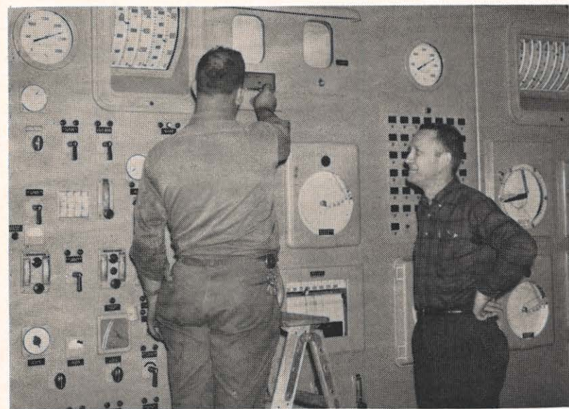
T. K. Skelton makes an adjustment on a closed circuit television control, while Mr. Painter observes. Maintenance jobs in a plant run from just delicate adjustments as this to repairing a chain-link fence.
