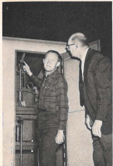
Mr. Painter and J. A. Moore, Glen Lyn plant manager, discuss a generator turning gear control.
