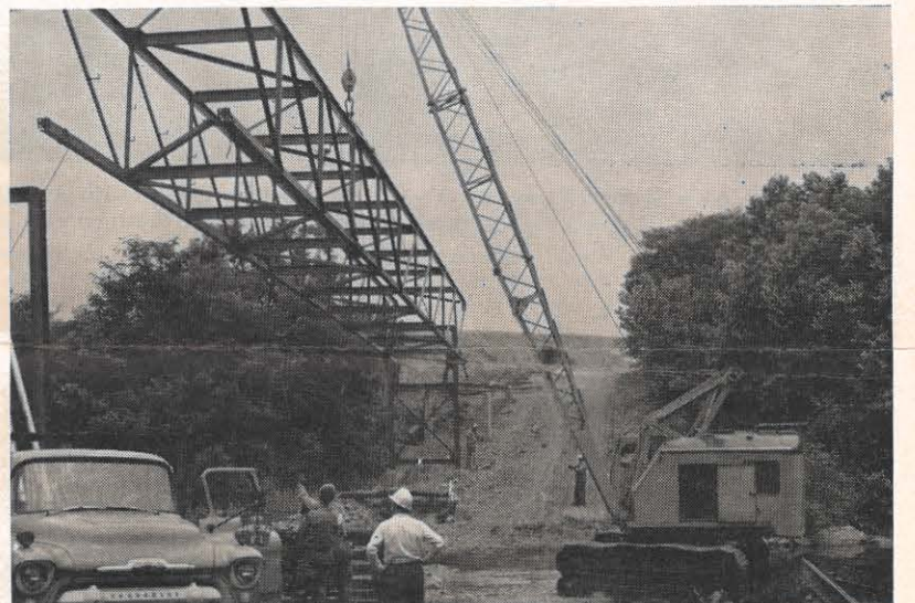
An overhead bridge, constructed by Glen Lyn plant maintenance men, will support ash lines running from the plant across East River to the ash storage basin. A section of the bridge is being lifted into place by the crane.
