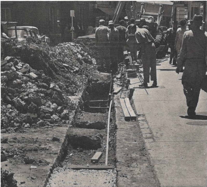
Appalachian has started a new underground project on Bluefield's Federal Street, at a cost of $32,000. The purpose is to permit sectionalizing of primary feeders to provide better continuity of service in the downtown area. Each transformer vault in the business area will have a means of switching from one circuit to another. The work will require three months.
