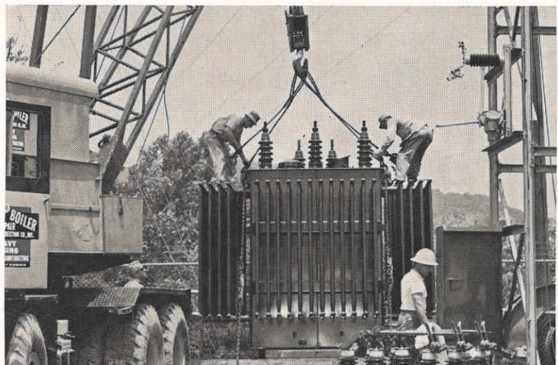
C. E. Yeager (white hard hat), engineer in the Huntington division, supervises the unloading of a new 3,750-kva transformer at Barboursville station. The new transformer doubled the capacity of the station, which serves an area whose demand is increasing at the rate of 11 per cent annually.
