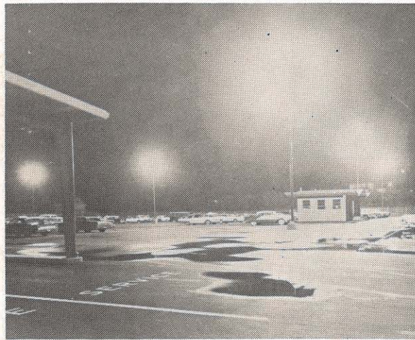
A new lighting installation, first on the Appalachian system, was used by Magic City Motor Corporation in its new quarters in Roanoke. Called The Powerglow, each of the five units in the area has a 224,000-lumen
