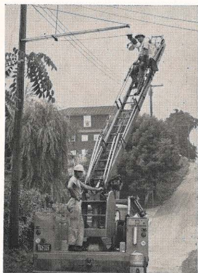
A pair of bulb snatchers at work. Street light attendant, J. T. Davis changes one of 3,300 lamps he is responsible for in the Lynchburg area. Helper, Fred Austin is at the bottom of the ladder.
