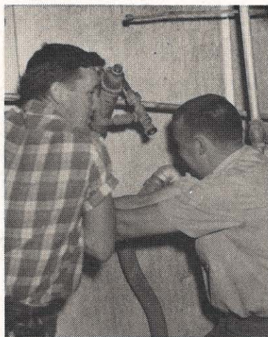
Instrument men Jesse Hackney (left) and Charles Low remove the boiler draft probes for repair.
