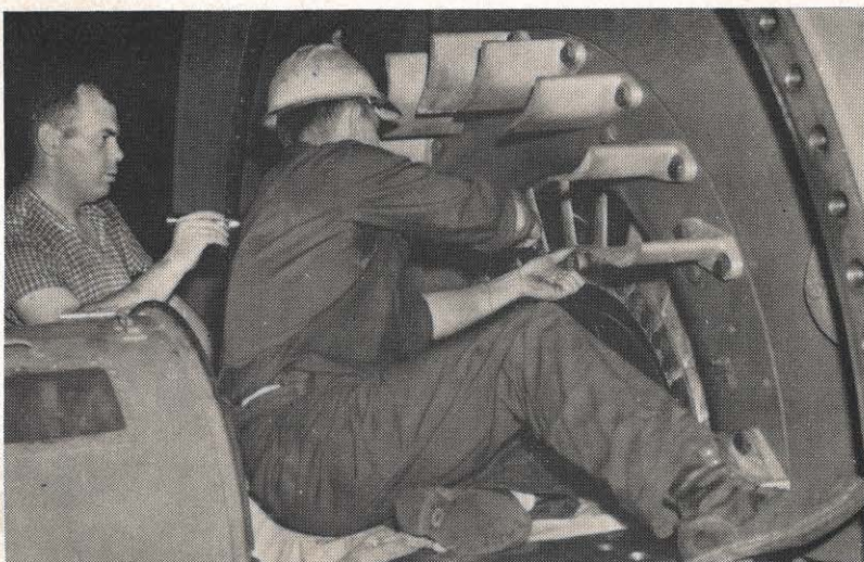
Marshall Stevenson (left) and Bently Grimes check the generator fan bolts for possible breakage.
