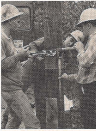
The affected areas are covered with fiberglass patches, and metal bands are wrapped around the pole.
