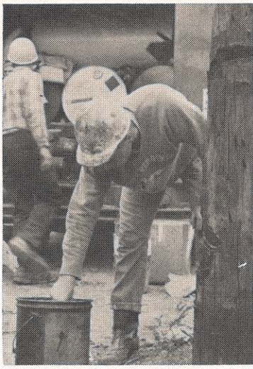
This pole has been examined and judged to be worth saving, in spite of deep cuts made apparent by a hatchet (top) and a roadscraper blade (left edge of pole), and the usual decay. Preservative is applied.
