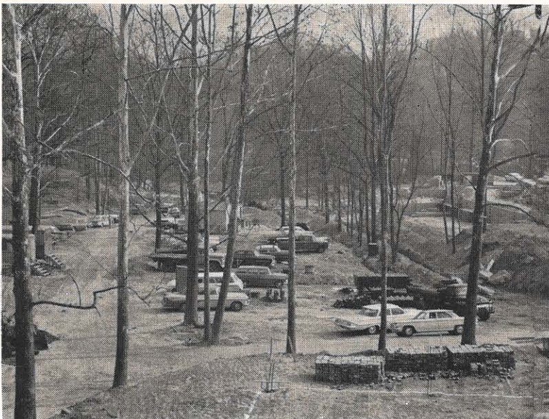
Charleston's third major total-electric apartment project, Greenbrier Gardens, is under construction. Electric service will be underground for the 30 buildings, covering 11½ acres in the South Hills area.
