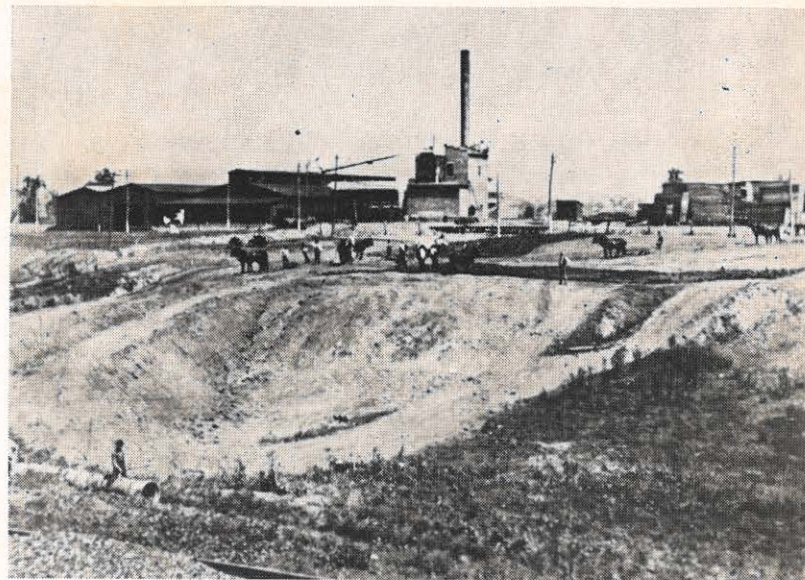
Theodore Roosevelt was president of the United States when this picture was made in 1903. It shows men and mules at work on the site of Kenova plant, being built by Ohio Valley Electric Railway Company.
