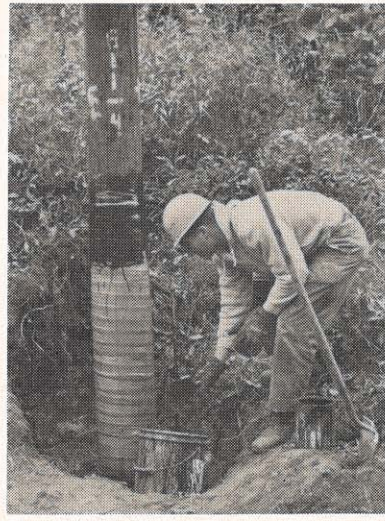
The sleeve now covers the pole and another layer of resin is applied. The total thickness of bandage and resin is about a half-inch.
