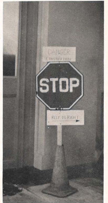
This sign in the Ashland office building is a real attention-getter. It warns office people of the opening in the floor for the new elevator shaft. Remodeling in the building is now nearing completion.
