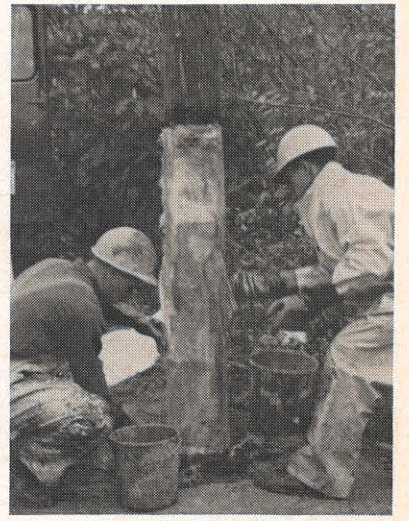
Bandaged and splinted, much like a broken leg, the pole now gets its final coat: a synthetic rubber compound to seal the wood from exposure to weather.
