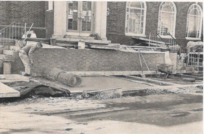
Heating cable goes into fresh concrete in the sidewalk in front of the Beckley office.
