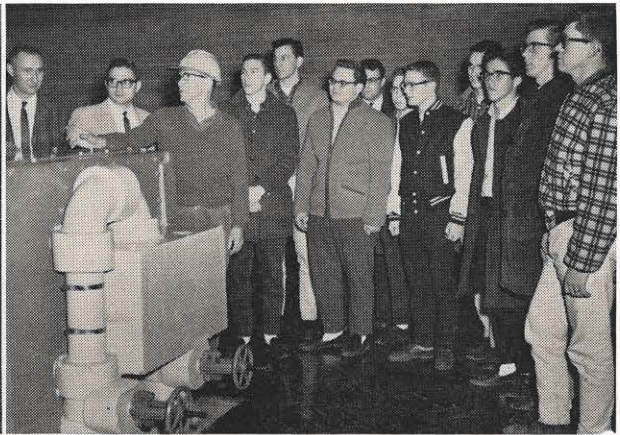
Business College. At right, the visitors from West Virginia Tech tour the London hydro plant, led by O. G. Harris, hydro operator.
