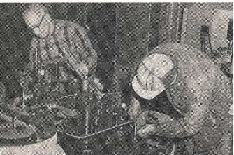
Clinch River's No. 3 unit was out of service last month for overhaul, inspection and cleaning. Boiler, boiler feed pump, high and low pressure turbines, turbine valves, ash hoppers, refractory, and preheaters all were looked after. Working here are W. A. Mitchell, General Electric field service engineer, and Con Powers, Clinch River master maintenance man.
