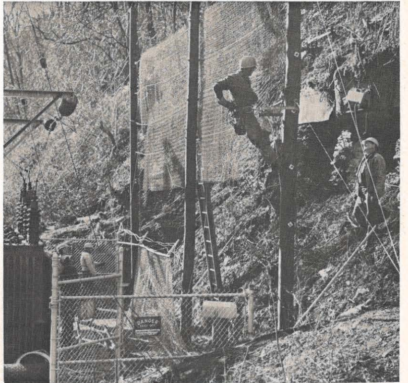
Brownwood station, near Beckley, has suffered damage in the past when rocks from the cliff above it loosened after freezing and thawing and rolled down into the structure. It won't happen again, hopefully, thanks to this barricade designed by the engineering group, and installed by L. C. Mollohan's station crew.
