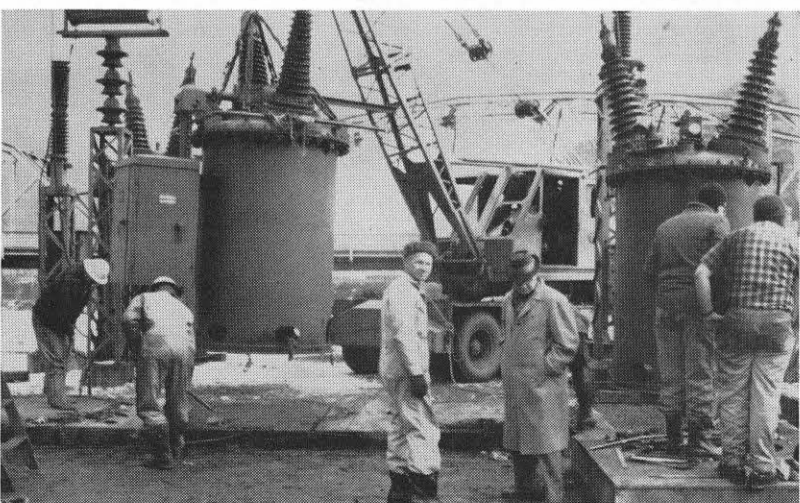
Logan employees raise the 138,000 volt breakers as part of the flood protection program being carried out in the Logan station yard.
