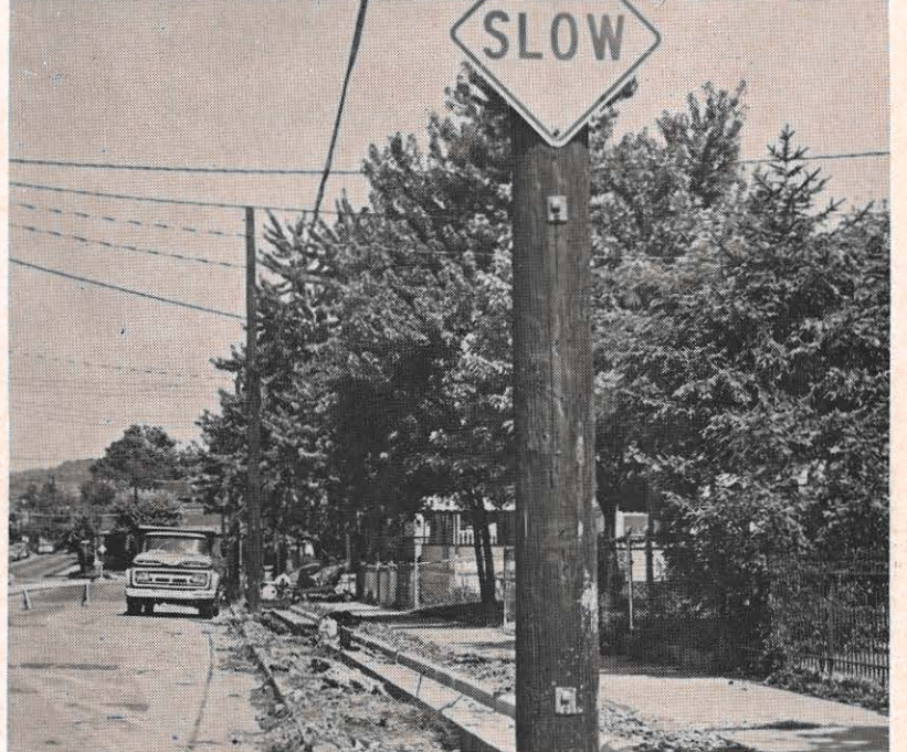
Where you have street widenings, there you have pole relocations. There is a lot of this work going on in Charleston, of which this photograph shows some. The construction of Interstate 64 requires relocating 128 poles in and around Dunbar. This picture was made of the 7th Avenue work in Charleston. (Daily Mail photo.)
