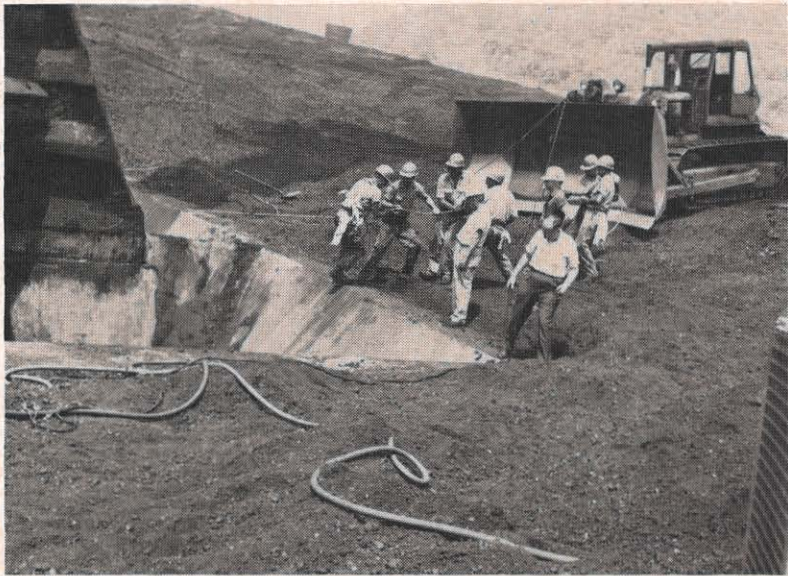
As part of the outage of Clinch River plant's No. 1 unit, much inspection work was done at the base of the standpipe and station hopper in the coal yard by the yard department. Other work done during the outage included the inspection of the generator, relining the ash hoppers, replacing cooler piping and rodding out condenser tubes.
