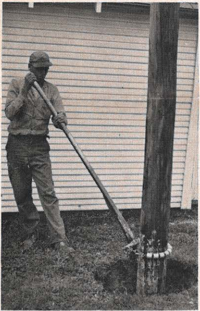
A new pole treatment, above, has started in the Roanoke division. It is called the Cobra Salts Treatment, and involves injecting a fluid mixture into the pole at ground level, and at regular intervals around its circumference. The holes are sealed with tar and the ground filled in.
