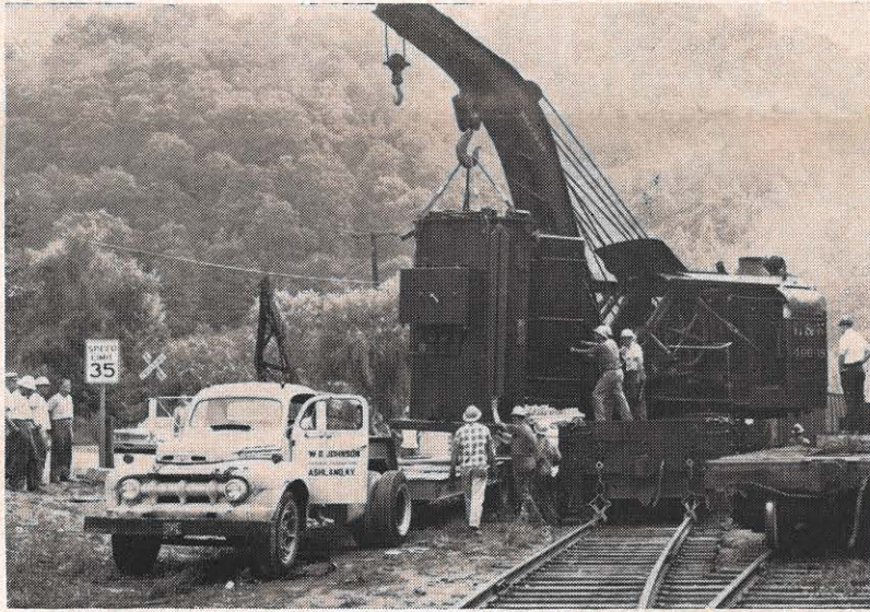
It's big, but it needs delicate handling. This is a 5,000-kva transformer being unloaded from a railroad flat car for delivery to Hazard division's new Bulan station. Watching the work by the side of the highway at left are W. C. Haddix, station foreman; Gaine Stidham, Clark Hays, and Russell Muncy.
