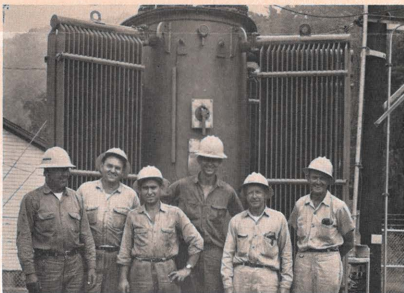
A new 3750-kva station has been put into service at Sharples in the Logan-Williamson division. It replaces a smaller station, and was made necessary by the steadily-increasing growth of coal mining operations. The Logan station crew is shown here by the new station; Siegel Hainor, Dallas Kinser, Jim Sullivan, Richard Trammell, Paul Adams, foreman, and Joe Pearl.
