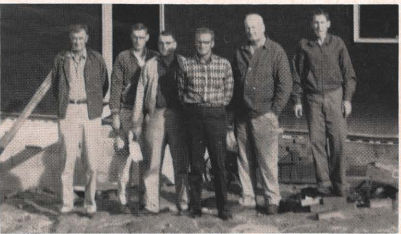
Ten Glen Lyn employees are pooling their time and talents to help build a parsonage for the Bozoo Christian Church. It's brick, seven rooms, and of course, electrically heated. The men are, from left, H. P. Jackson, L. B. Jackson, E. W. Ganoe, W. H. Dillow, J. C. Keatley, and R. K. McLaugherty. Others working on the project but absent from the picture are T. B. Skelton, H. Jackson Jr., D. T. Hayner, and H. O. Brookman.
