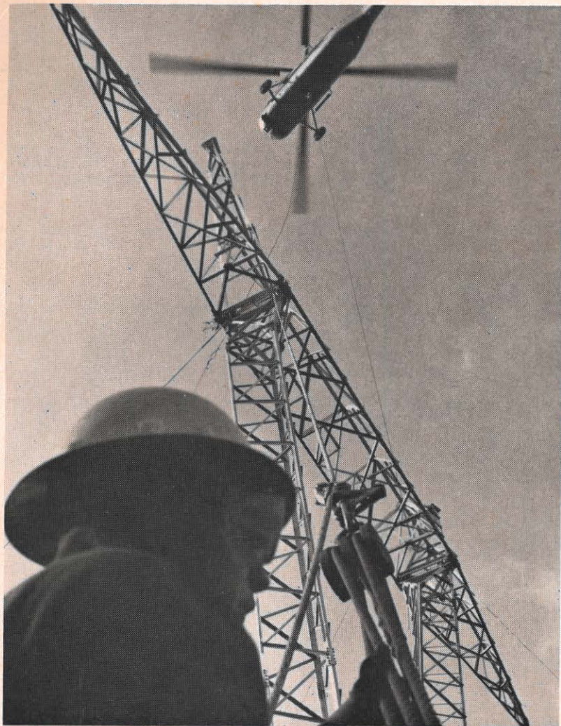
This was a typical scene of activity recently when helicopters began the job of lifting and setting aluminum V-shaped towers in the Sporn-Huntington 345-kv line. (Photo by Jack Burnett, Huntington Publishing Company.)
