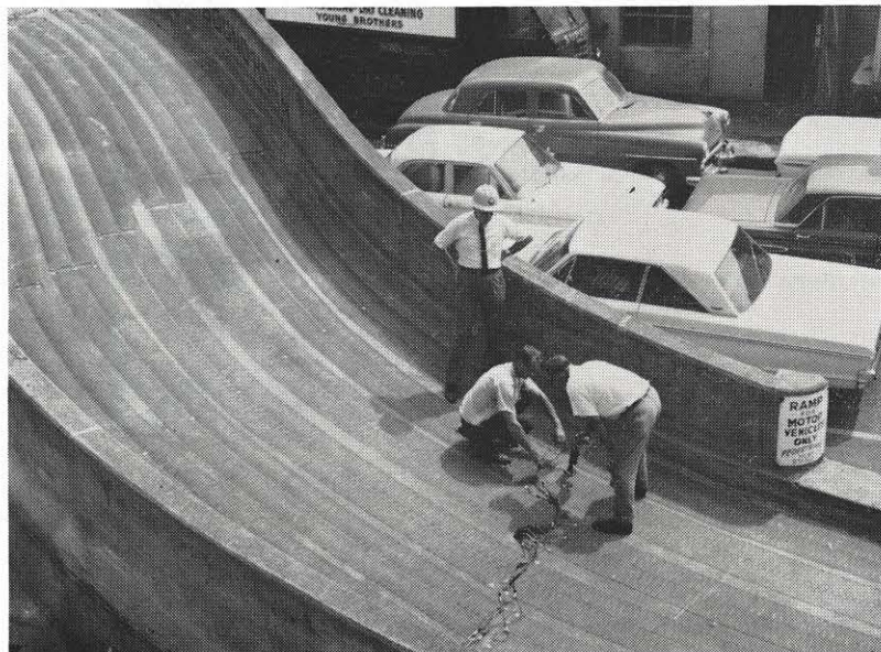
Jim Crane, standing, building service supervisor in Charleston, watches the installation of wire which will deliver heat to 30 mats in the ramp leading to the second deck of the Virginia Street garage. A layer of blacktop will be rolled over the mats, and will, thanks to electricity, stay dry and safe in bad weather.
