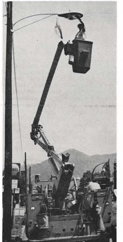
Bob Metz, area serviceman, completes the installation of a 21,000 lumen mercury vapor lamp in Montgomery in the Charleston division. W. D. Grimmatt and Mason Wood watch from the ground. Altogether 198 of the new mercury vapor lamps were installed to replace the town's old incandescent lights.
