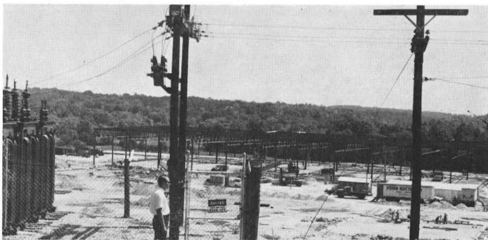
Industry is power: Joe Higgins of the Fieldale area office stands by a temporary station built by Appalachian to serve the U. S. Gypsum plant under construction near Danville.
