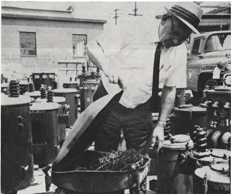
A transformer recently taken out of service in Abingdon was found to be doing double duty. Apparently a corner clamp came loose, and opened the top sufficiently to allow birds to enter and set up housekeeping for their young. Lloyd Smith, stores supervisor, above, found about a gallon of straw in the transformer.
