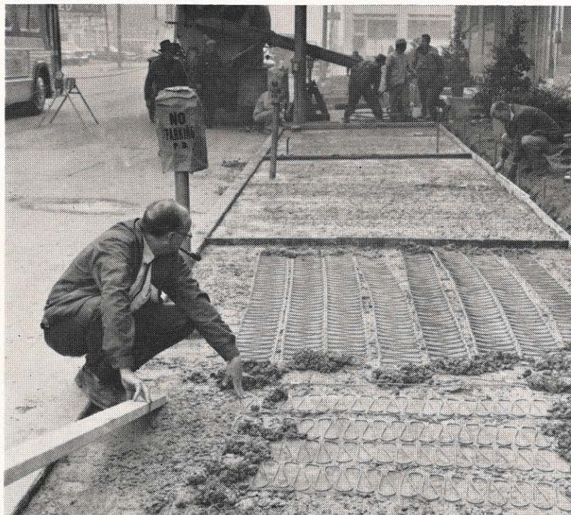
Four hundred feet of new sidewalk around the Charleston office building will be dry when the snow begins to fall. Jim Crane, building supervisor, inspects the repaving work. A special sensing device mounted on the building roof will automatically cut on the thawing equipment at a given point of temperature and relative humidity.
