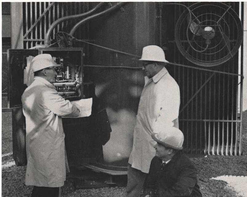
Ed Yeager, Ted Smith, and Oscar Fowler, give a 34.5-kv transformer a final checkout before energizing it in Huntington. The equipment is part of the Fulks downtown station, which serves Marshall University's seven-story, all-electric classroom building, now nearing completion.
