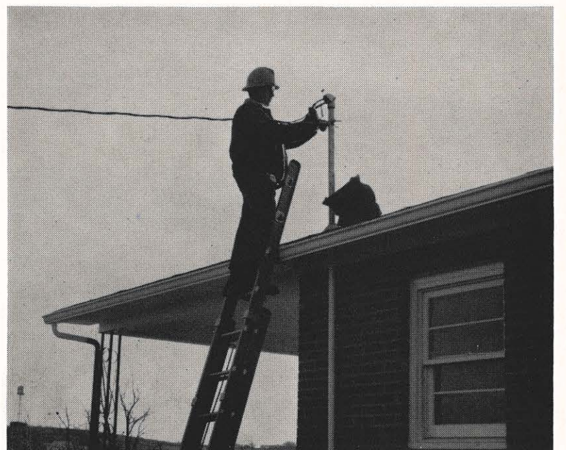
Symbolizing the increasing use of power in the Pulaski division is this picture showing a service connection by W. P. Brewer Jr., of the division service crew. Average annual residential usage in the division has now passed 6,000-kwh.
