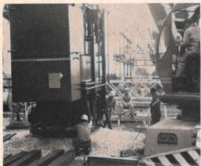
Kentucky Power's Ashland division recently came upon the problem of transferring a 92,100-pound transformer from one site to another. It was solved by the use of two cranes, 40- and 35-tonners, that set the transformer on a low-boy which hauled it to the substation. Using this procedure, only six hours were required to finish the job.
