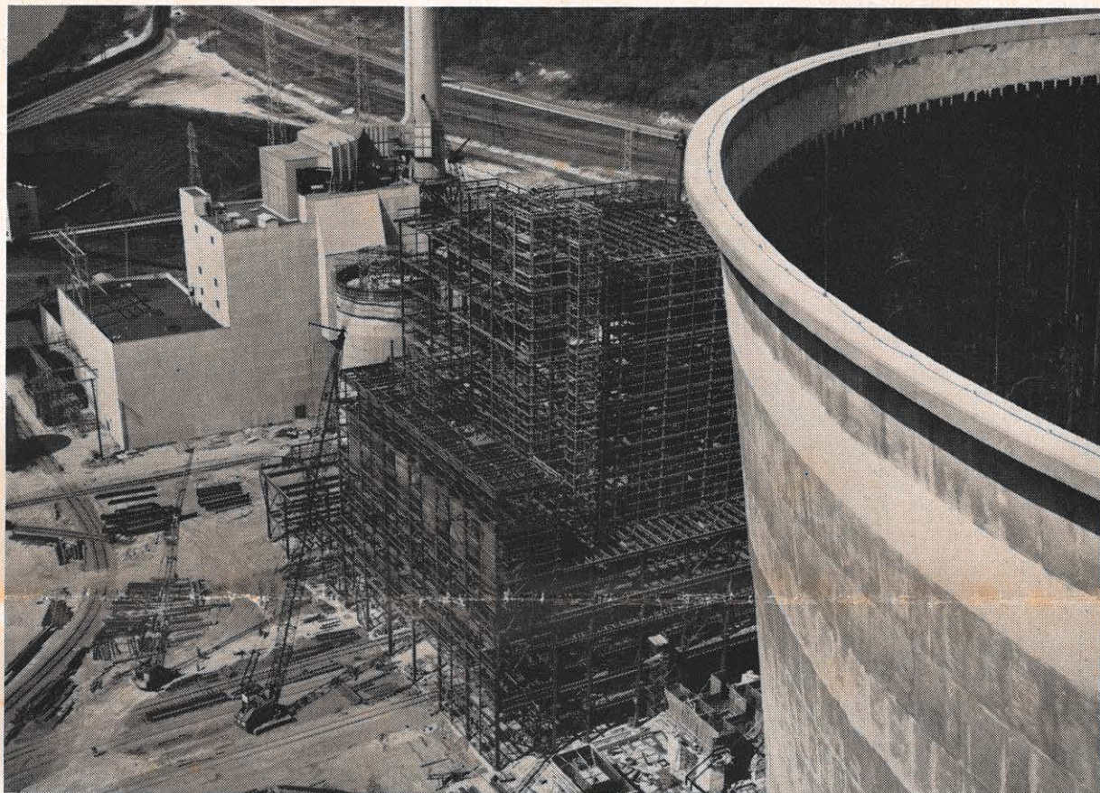
The new cooling tower at Kentucky Power's Big Sandy Plant shows the construction area for the plant addition and the existing plant in the background. This
