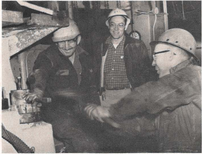
Clinch River's Lewis Kenney, Page Ott and Giles Carter (left to right) tighten cover on boiler feed pump turbine H-P stop valve.
