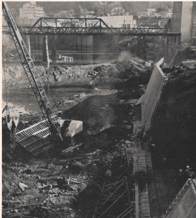
In 1963 and again in March of this year, flood waters in the Logan area caused extensive damage to the retaining wall at the Logan switchyard. Presently workmen are making repairs behind a dike which is diverting the river so that the men can work eight feet below the normal water level.
