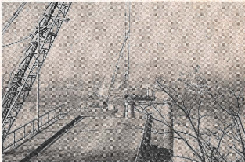
Approach to the fallen bridge.
