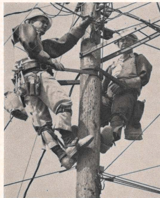
F. E. Austin (left) and S. L. Drumheller are linemen in the T&D department, Lynchburg division. Their main job is making sure the electricity we provide gets to the customer's home. If it isn't there when the switch is turned on, our dependability might be questioned. These are some of the men who make sure it is there.
