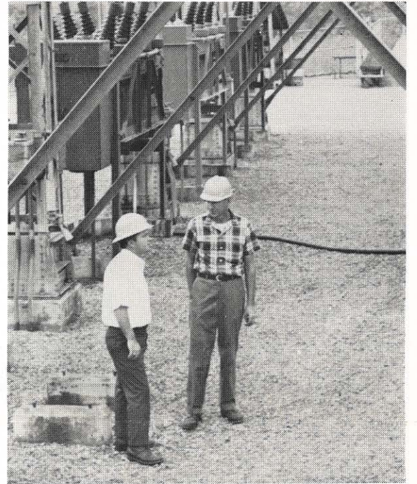
G. L. Elden, station foreman, and Wooten check station for unsafe conditions.
