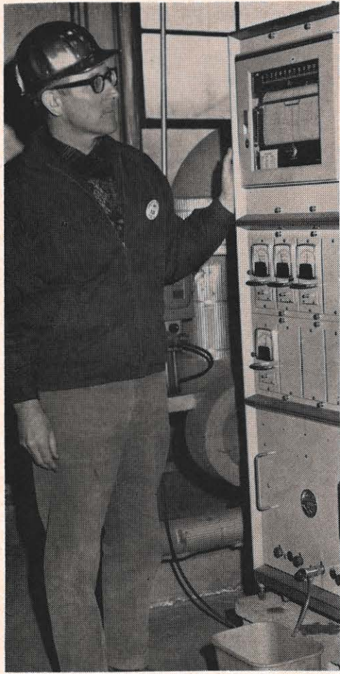
Miskimen checks river monitoring device at Kentucky Power's Big Sandy Plant. This raw water monitor was installed for the Kentucky Water Pollution Control Commission and checks raw river water for the following conditions: river temperature, dissolved oxygen, PH and conductivity.
