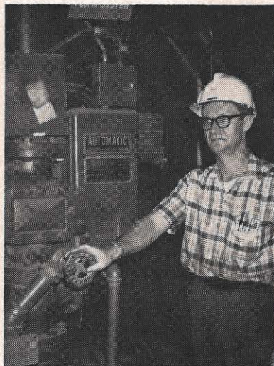
Fire Marshal Lovell H. McDonald check out the Unit No. 1 basement foam system. This system is very important to fire protection in the plant.
