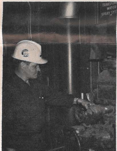
Brigade Captain Alvie Napier inspects one of the transformer water spray systems at the plant.
