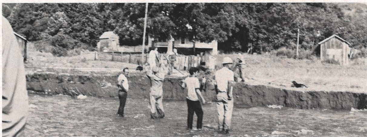
Appalachian linemen restore service to home in Nelson County as local volunteers go about other duties.
