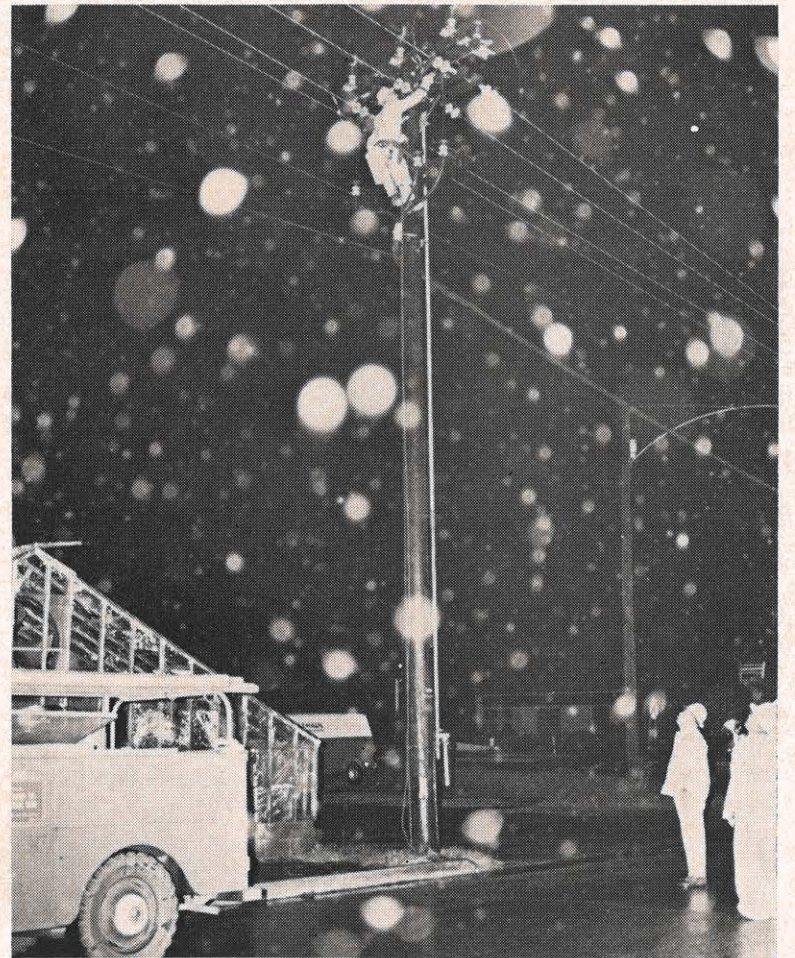
Winds up to 56 mph and heavy rains brought down trees and lines throughout the Teays Valley-St. Albans area August 9. Line crews were kept busy throughout the night answering scattered calls and restoring service. Here near the Nitro Bridge, members of one crew watch as an Appalachian lineman reconnects lines blown down during the severe storm.
