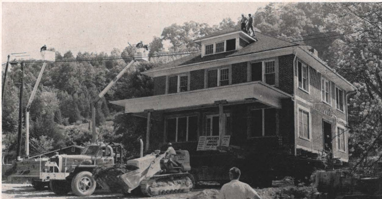
This brick home, one of the oldest and largest in Pike County, had to be moved from the path of the new highway replacing U. S. 23 and 460. Pikeville crews raised the lines and the house was slipped under so that service to several area customers would not be interrupted.
