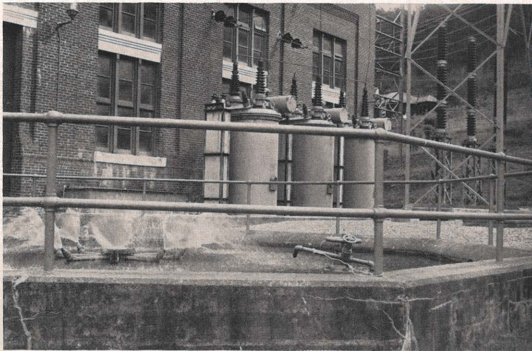
Water is fed to the cooling pool from a mountain spring. This is the last of the "water cooling systems" to be employed by Appalachian.
