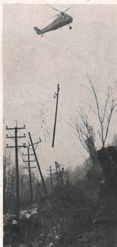
Roanoke Division is rebuilding part of the 34.5 kv arterial system through the heart of the city. The project involves 12 miles of line, 215 poles and 16 months of construction.
