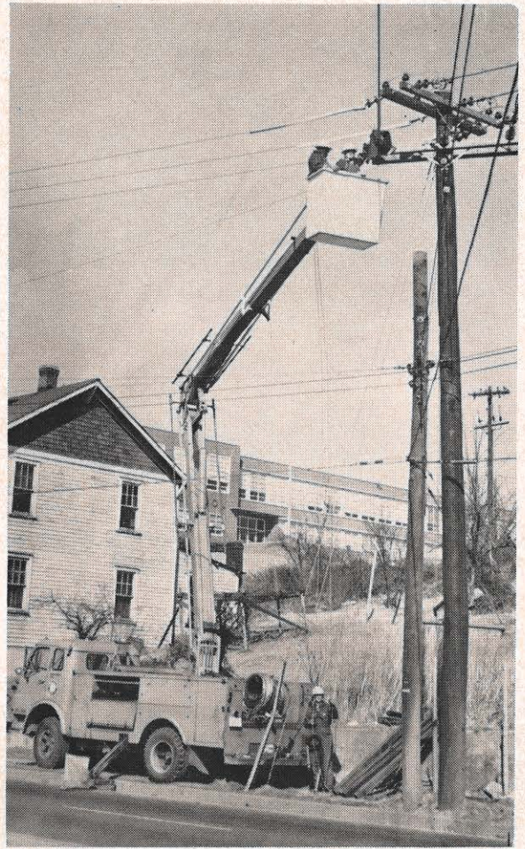
A common site throughout the AEP System is a line crew using a bucket truck. Our system is among the first in the nation to use extra wide flotation tires for improved operation. Here L. S. Caldwell and John McManway (both in the bucket) and C. W. Hodges make repairs in Roanoke.
