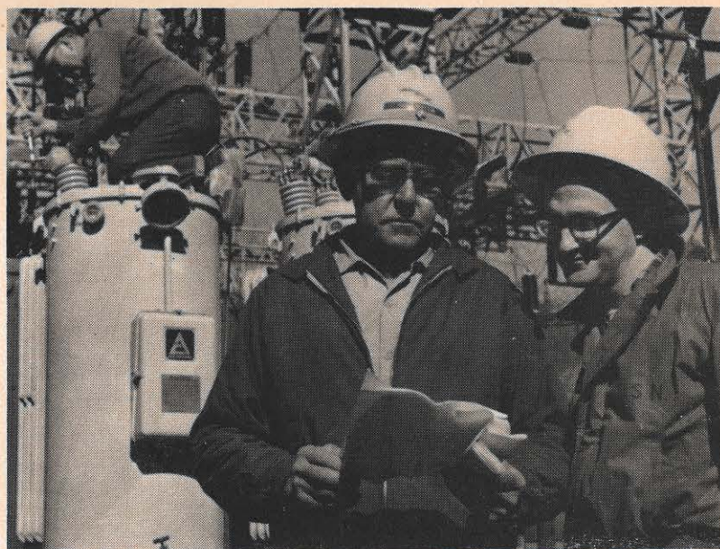
Hansel Stratton (front, left), line foreman, discusses the job print for installation of voltage regulators at the Coalton Station with Chris. In the background is John Cornette, lineman A, working on the new regulators.
