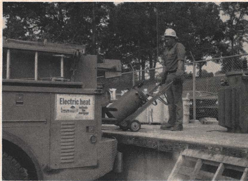
D. R. Woolwine, lineman A, loads the transformer that is to be used for the service.
