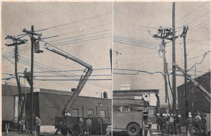
Bucket truck (left) is used to secure hot lines to arm on temporary pole at the same time the telephone cables are being attached to pole. The new pole is placed in the exact same spot (right).
