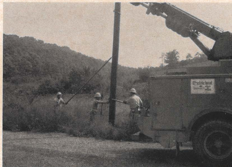
Setting the pole in place is (left to right) Clayborne Wirt, Kenith Dawson, lineman C, and Raymond Profitt, truck driver-groundman. Then the lines are installed and the meter placed on the house.
