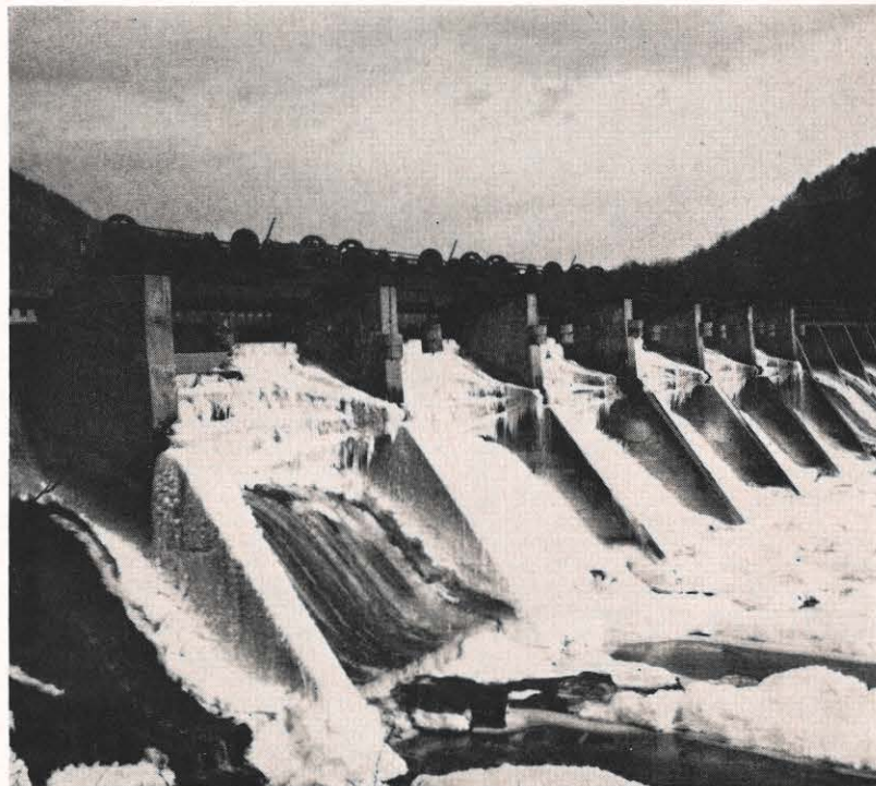
Ice built up on the taintor gates when water overflowed the spillway at Buck Hydro Plant on New River, Pulaski Division, during the recent cold weather. The overflow was caused when mush ice blocked the flow of water to the turbines and thus shut down the generators.
