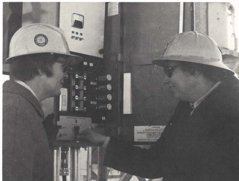
Janet Wynot, left, watches as Helen Young closes the circuit to energize the Bent Mountain Station.
