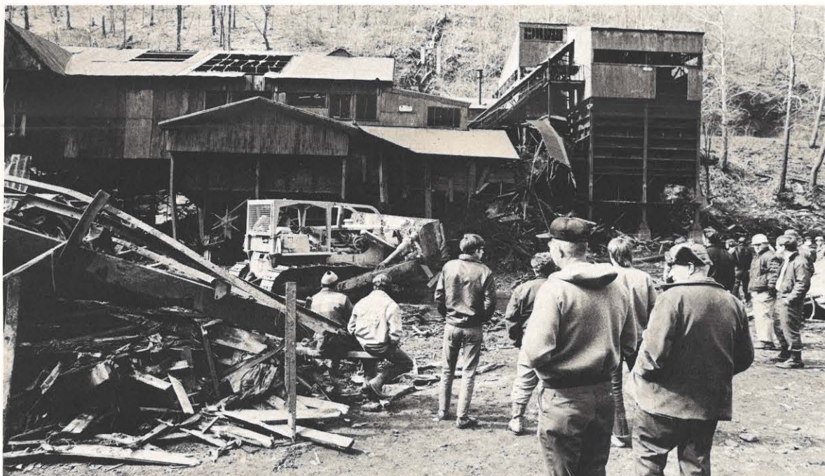
Cleanup operations begin at the processing plant of the old Lorado Coal Company, located about one-half mile upstream from Lorado. Photo courtesy Huntington Publishing Company.
