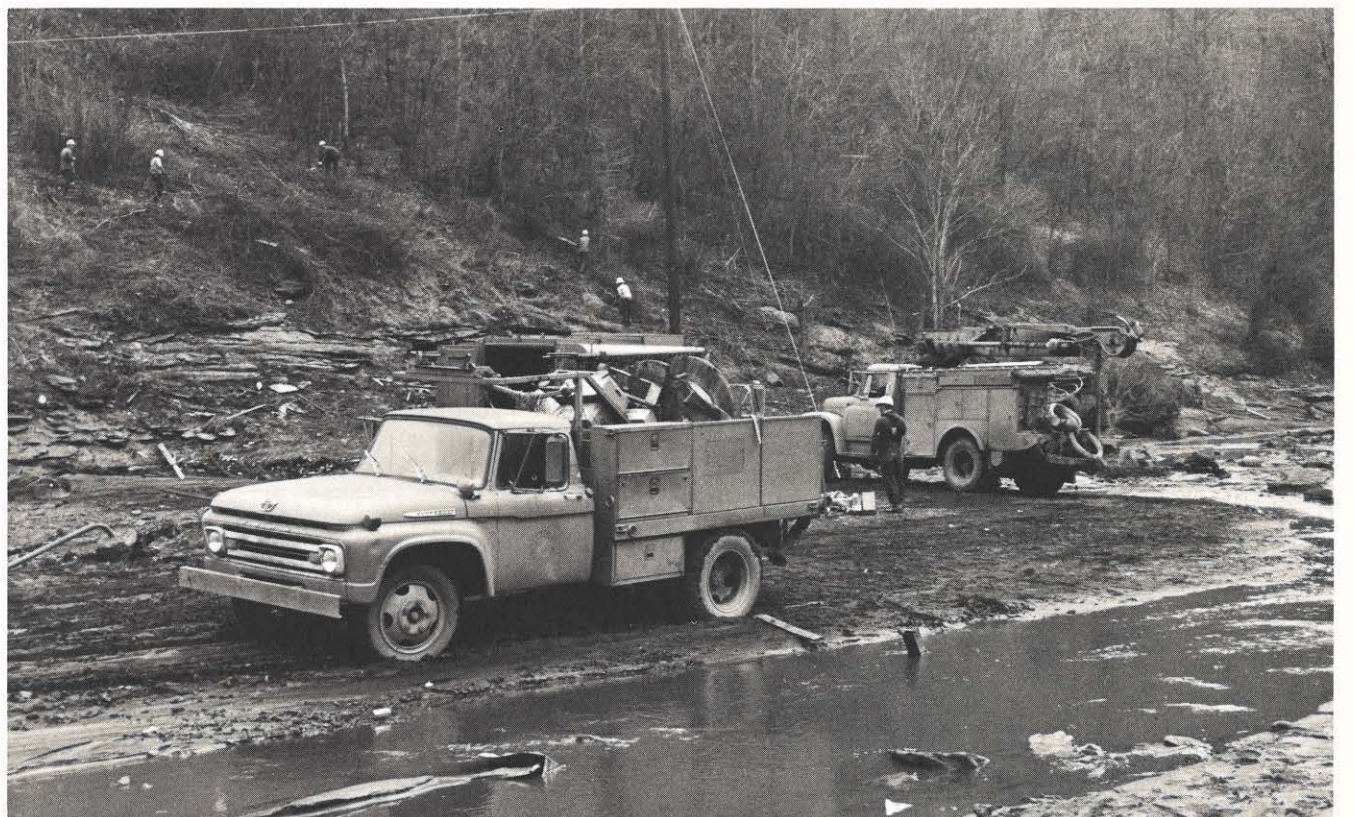
Employees working to build a new line in the Pardee section of Buffalo Creek.
