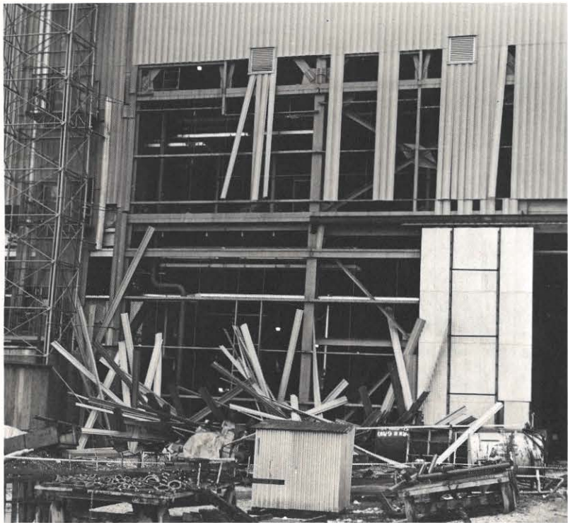
28 CONSTRUCTION WORKERS were injured, none seriously, in an explosion March 2 in the elevator pit of Unit No. 3 under construction at the John E. Amos Plant. A section of the outside wall, approximately 40 feet x 40 feet, was blown out and the shaft on the interior of the building was extensively damaged. Evidence indicates mapp gas leakage from a cutting torch collected in the elevator pit and ignited, causing the explosion.
