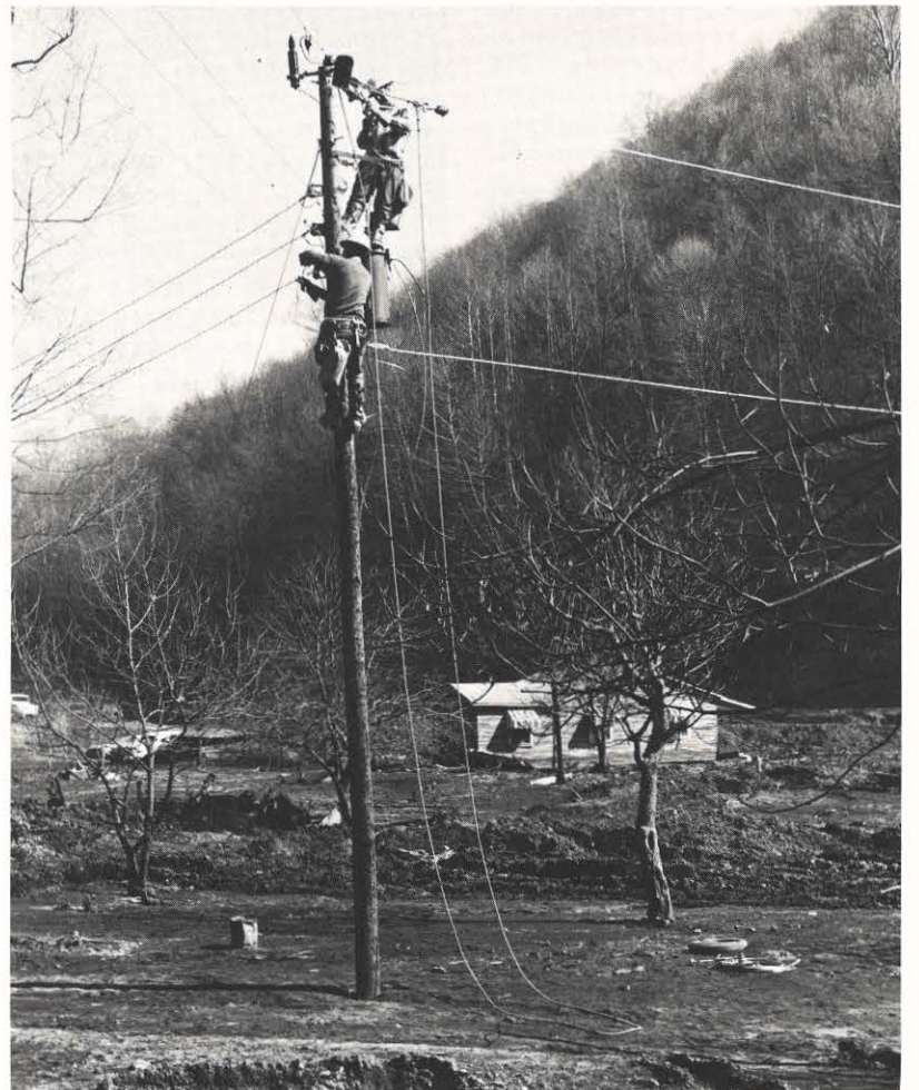
Appalachian employees restore service to the one remaining house in the second camp of Robinette, West Virginia.
