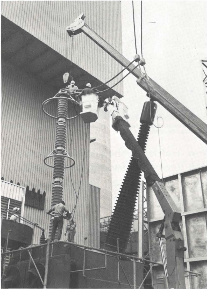
Members of the General Office T&D high line crew out of Charleston, headed by Frank Harmon, install the conductor on top of a new lightning arrester at John E. Amos Plant. During a severe electrical storm July 11, the old lightning arrester literally disintegrated, knocking out Unit 1.
