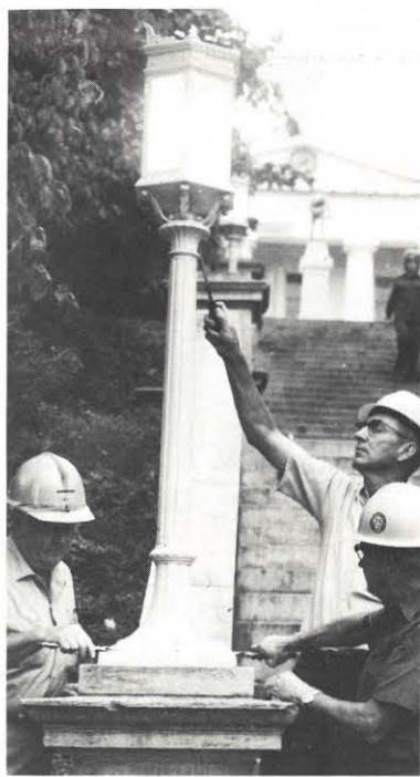
Installing the newly painted light standards are (l. to r.) D. E. Booth, stationman A; G. E. Elder, station foreman; and S. S. Gilbert, stationman A.
