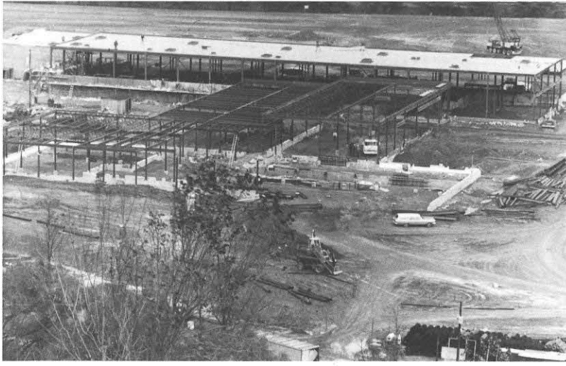
CONSTRUCTION of the Roanoke Service Center is 30% completed. The $3.2-million project began in June, shortly before Hurricane Agnes swept through Roanoke. The entire 44-acre tract on which the Center is located was flooded. Large amounts of fill dirt was brought in to raise the elevation of all this project above the high water mark of 918.7 feet above sea level. A target date for completion of the service center has not been set.
