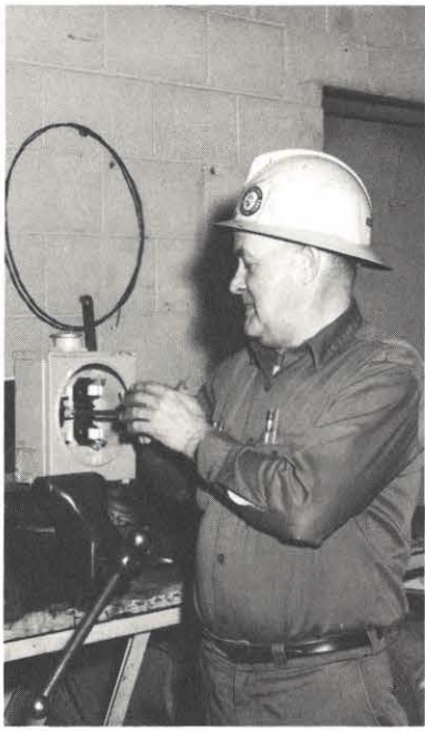
C. H. McVey prepares a meter base for installation in the Tazewell area.
