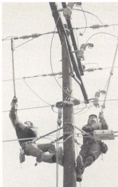
A. J. Parsons (left), lineman B, and E. B. Suthers, line foreman NE., energize line as 34.5 kv for the first time.
