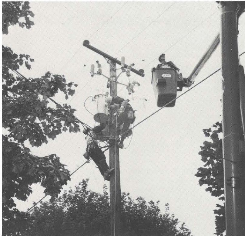
On schedule is the conversion of Smyth County, Va. to 34,500 volt distribution. Here, a Marion line crew completes the installation of a 34,500 volt transformer bank near Chilhowie.
