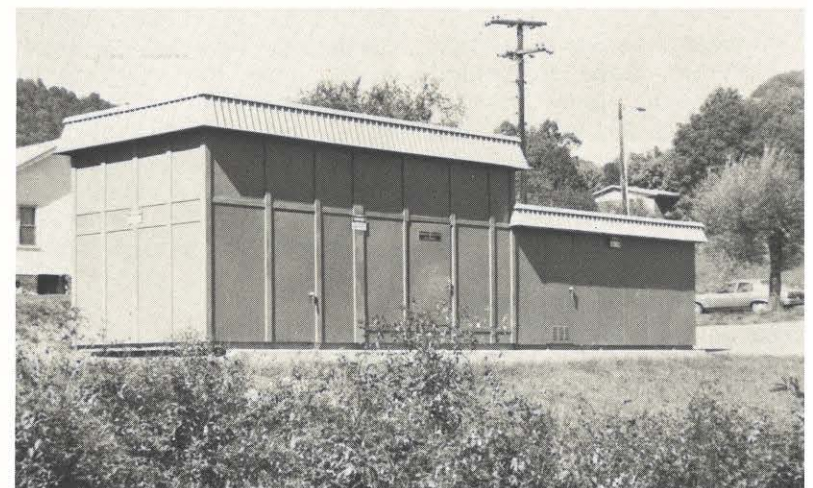
This 69 kv modular station at Weber City in Abingdon Division is the first in Appalachian Power's System.
