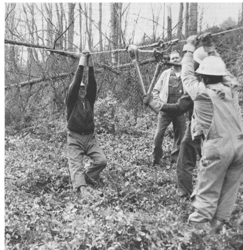
A Rocky Mount crew (Roanoke Division) makes repairs to a single-phase line paralleling Route 40 west of Ferrum to get the line back in service.
