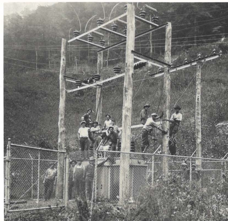
This photo was made during the construction of the Pond Substation in the Madison area of Logan-Williamson Division. Note the absence of hard hats.
