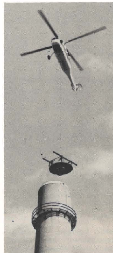
A helicopter removes the scaffold from inside the stack liner of Philip Sporn Plant Unit 5.
